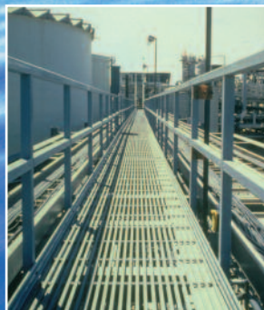
Personnel walkway, chemical and waste water treatment plants.
