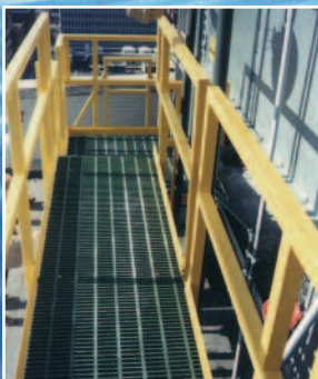
Cooling Tower featuring Seasafe grating and handrails.
